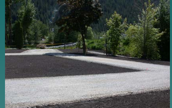
Backfill complete, sod or grass seed will be placed on soil areas.
