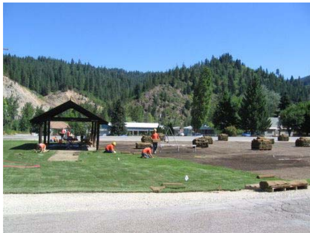
Workers lay down fresh sod, wrapping up clean up of Lion's Park in Osburn.
