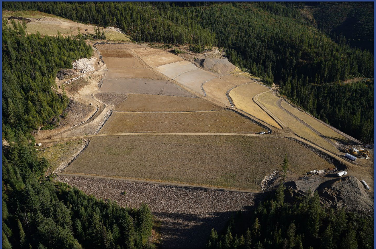
East Fork Ninemile Waste Consolidation Area. Images provided by the CDA Trust.
