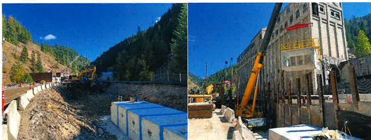
Box culvert install in Canyon Creek. Images provided by the CDA Trust.
