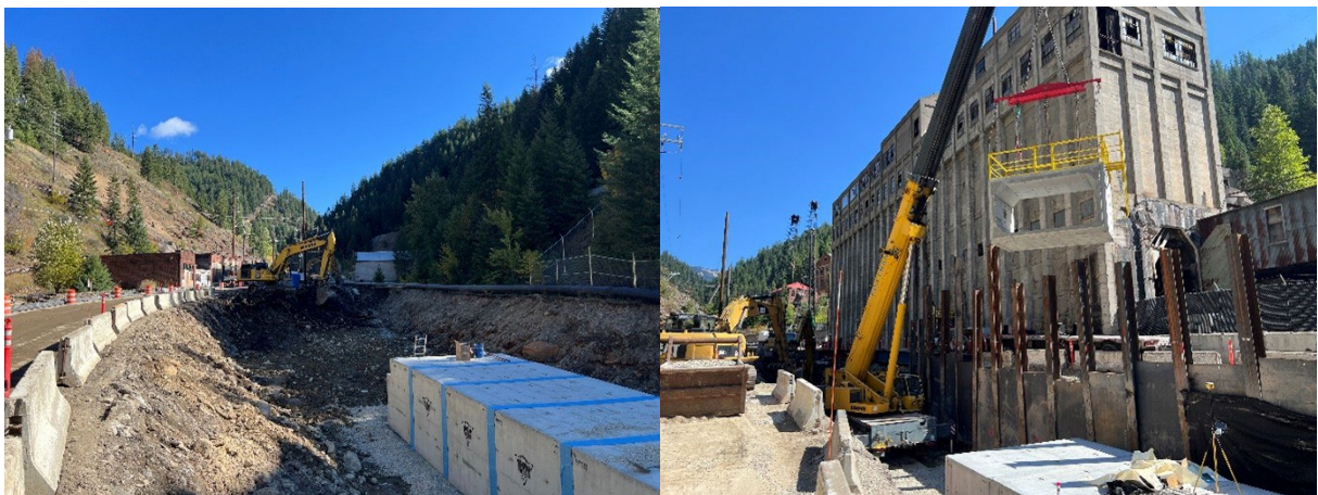
Box culvert install in Canyon Creek. Images provided by the CDA Trust.
