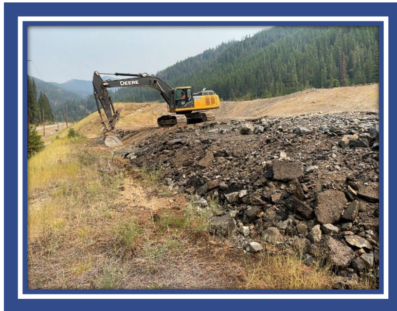
Lower Burke Canyon Repository waste grading. Image provided by the CDA Trust.
