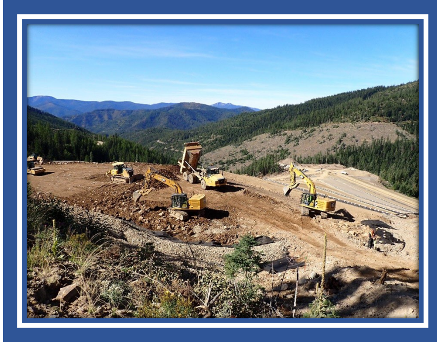
East Fork Ninemile Waste Consolidation Area waste placement. Image provided by the CDA Trust.
