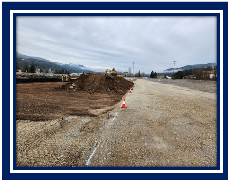
Facing west showing excavation of top foot of contaminated soil along south edge of Theater Bridge Road. Photo courtesy of Idaho Department of Environmental Quality.
